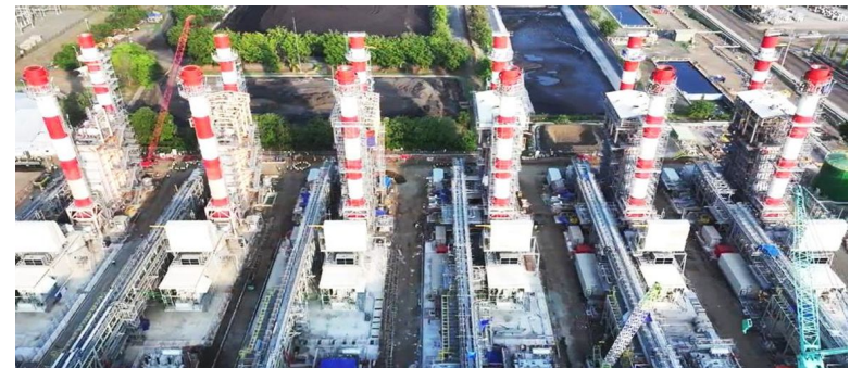
Gas and Steam Power Plant
